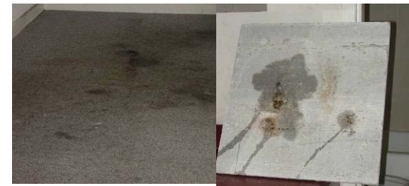
Commissioning / Operational Issues Humidity & Mold
